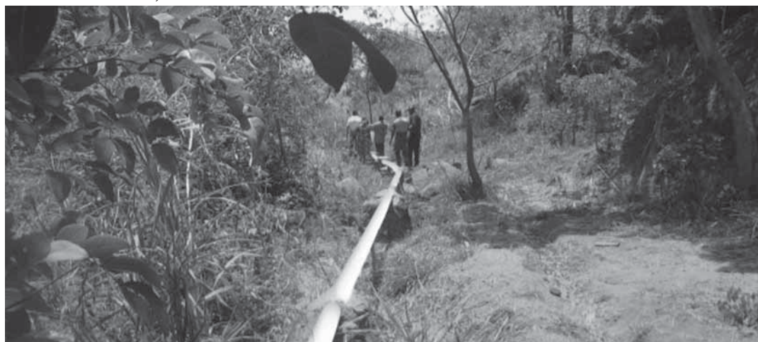
A pipeline channeling water for domestic use and irrigation
