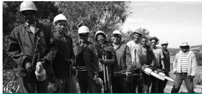
South Africa. Clearing invasive alien plants from waterways is part of Overstrand Municipality's comprehensive water management strategy, and has provided jobs and training to thousands of people. Source: Overstrand Municipality
