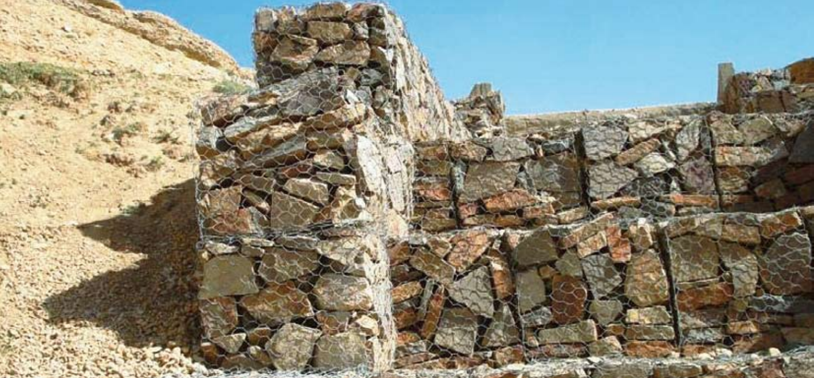
Gabions are large metal boxes/cages, which can be filled with stone and/or gravel and placed on riverbanks and other locations to work as flood-resistant walls. (Photo courtesy of IRIN News)
