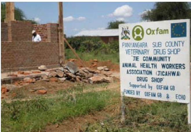
Inspecting ongoing work for the animal drug store construction in the community (Photo courtesy of Oxfam GB)
