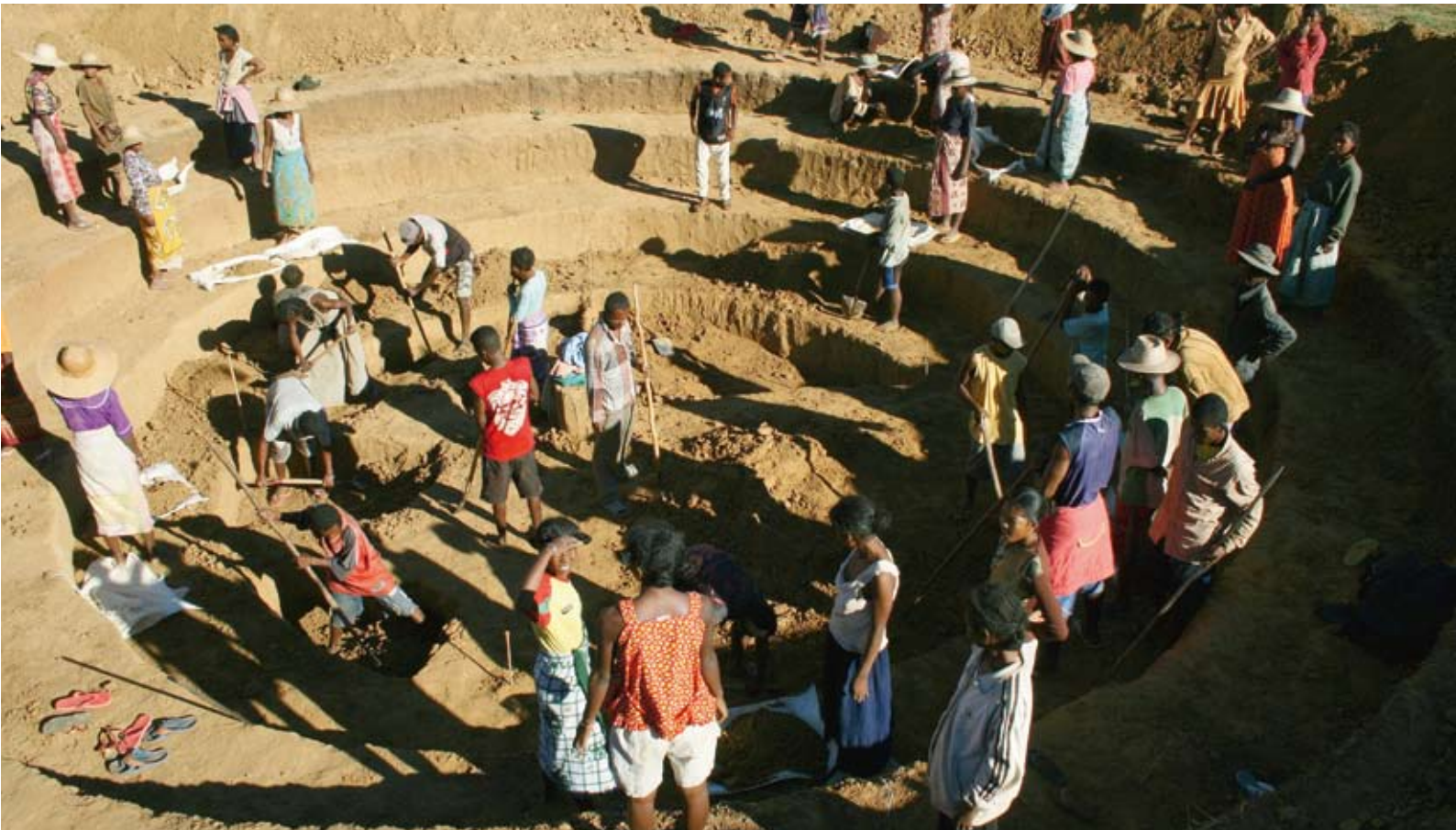
A community near Ifotaka, in southern Madagascar, pulls together to build a rain water harvester. (Photo courtesy of IRIN news)
