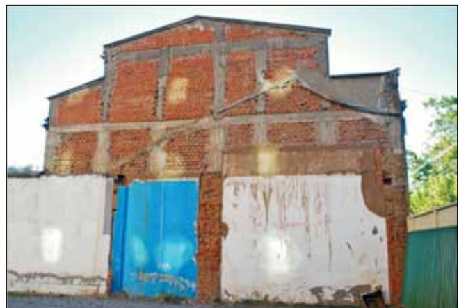
FIGURE 13. Examples of the typical performance of unreinforced masonry buildings in Chile (heavy damage and collapses) and confined masonry buildings (usually only lightly undamaged) in some of the most damaged towns in the 2010 M8.8 earthquake buildings.
