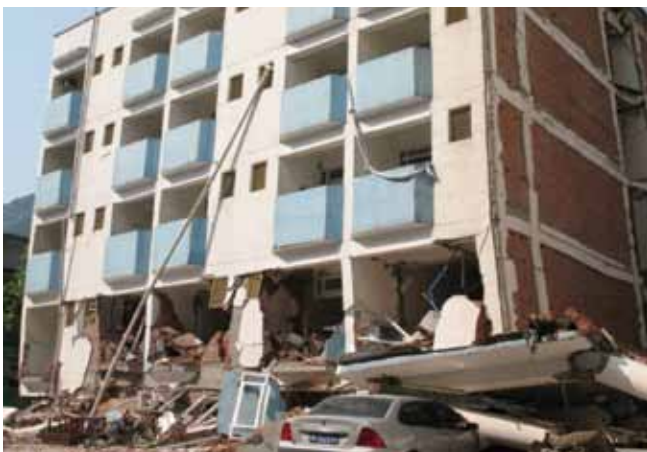
FIGURE 6. Collapsed ground floor of a hospital building in Mianzhu, 2009 M8 Sichuan, China earthquake.
