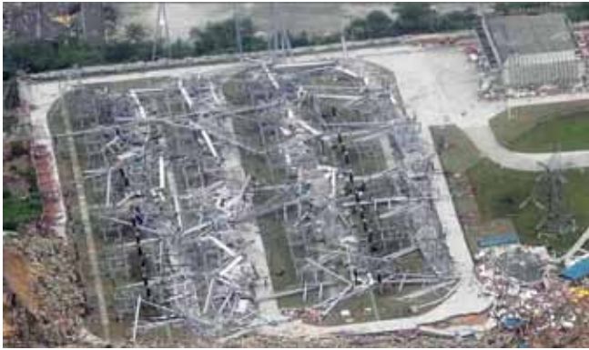
FIGURE 4. Near total destruction of the 220 kV Ertaihan Substation, Yingzhou in the 2009 M8 Sichuan, China earthquake.
