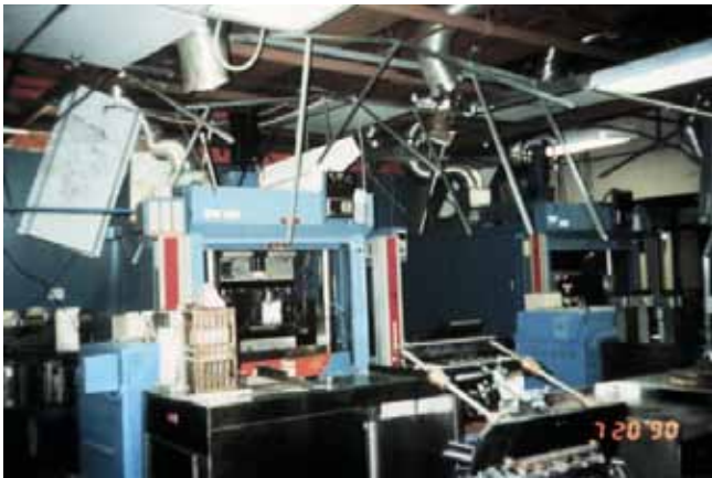
FIGURE 2. Damage to unprotected equipment and non-structural items in a clean room of an electronic components assembly plant, Baguio, Philippines, 1990 M7.7 earthquake. The building itself was not damaged significantly. The equipment damage caused a 3-month long business interruption and a major financial loss.
