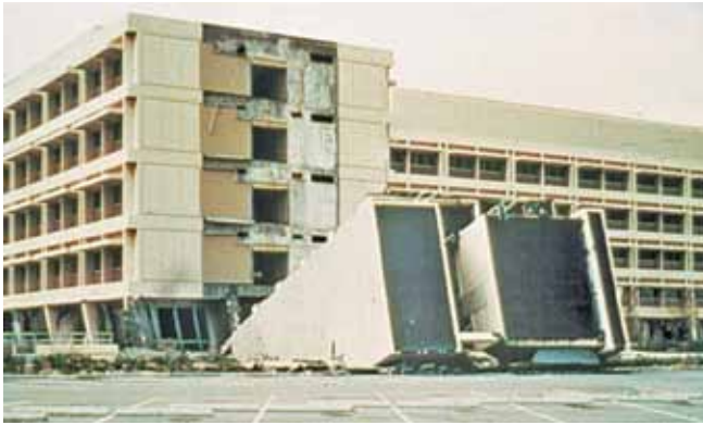
FIGURE 7. The collapsed three month old main building of the Olive View Hospital, San Fernando (Los Angeles, California) M6.7 earthquake of 1971.
