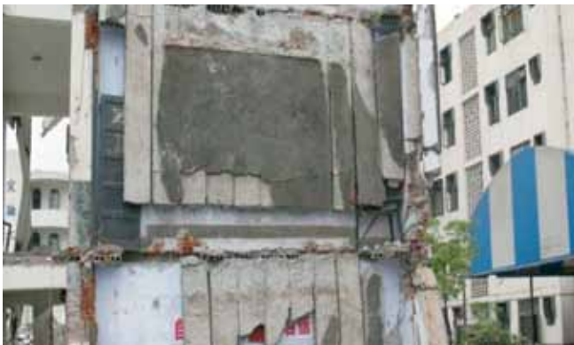
FIGURE 5. Partial view of the interior of three vertically stacked school rooms in a collapsed middle school in Dujiangyan; 2009 M8 Sichuan, China earthquake.
