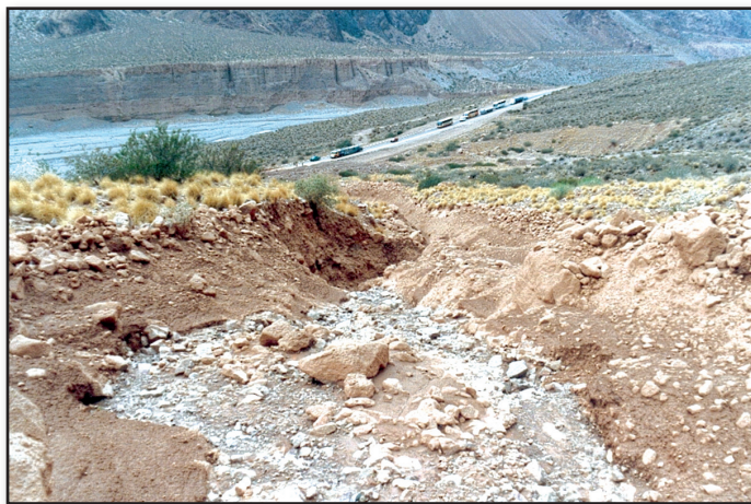
SEVERE EROSION OF SLOPES THREATENS THE ANDEAN CORRIDOR AND THE RIVER.
