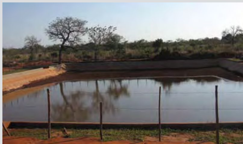
Through an OFDA-funded project, community members worked together to build a water catchment area in Liozuane, Mozambique. The completed reservoir is nearly the size of an Olympic swimming pool (Top and center photos by Ian Moise, USAID; bottom photo courtesy of IRD).
