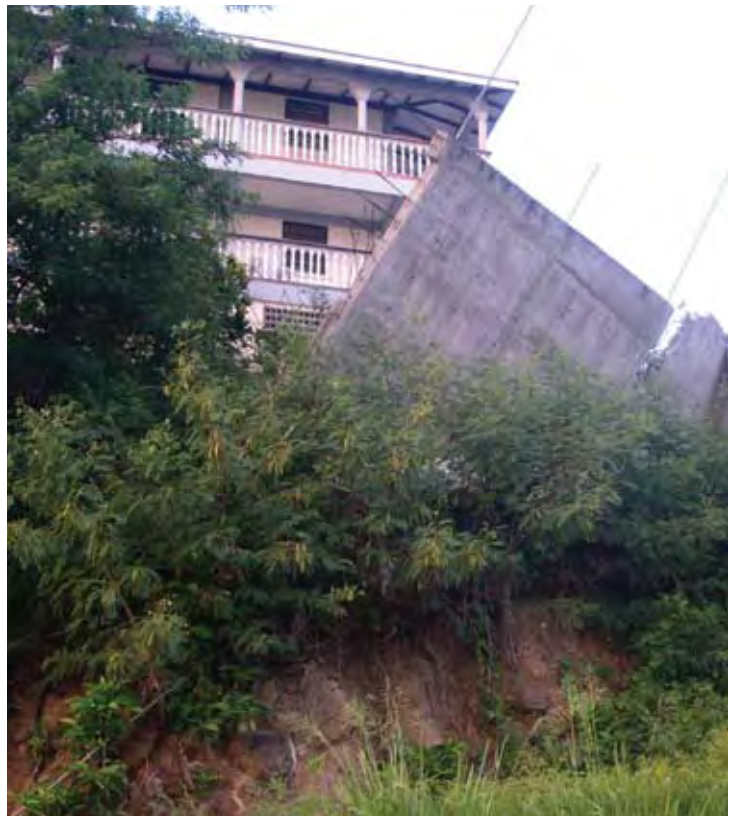
A large slab of concrete from a damaged building rests precariously on a hilltop in Dominica following Hurricane Dean (Photo by Julie Leonard, USAID).
