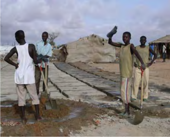
IDP youth construct latrine slabs in Kass, Sudan, as part of an OFDA-funded livelihoods program (Photo by Laura Chapman, USAID).
