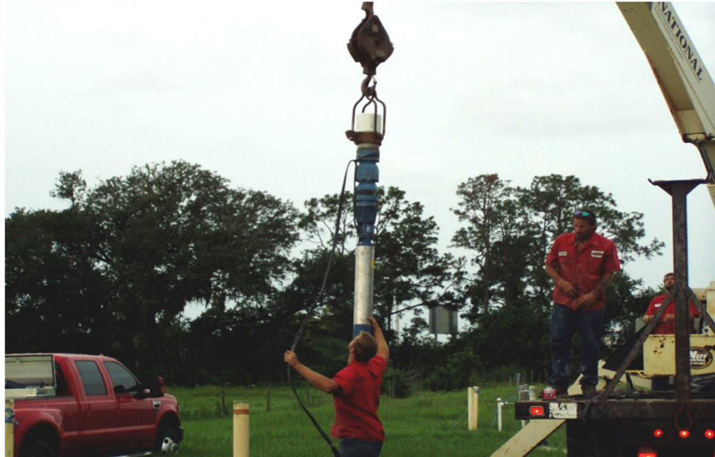
Figure 8. Pump installation at St. Cloud site.
