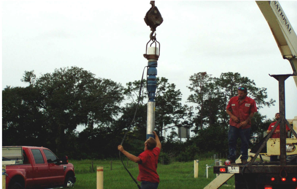
Figure 8. Pump installation at St. Cloud site.
