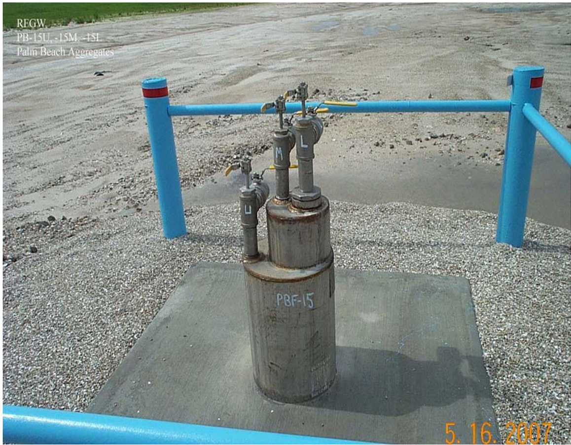
Figure 4. Photograph of PBF-15 wellhead.
