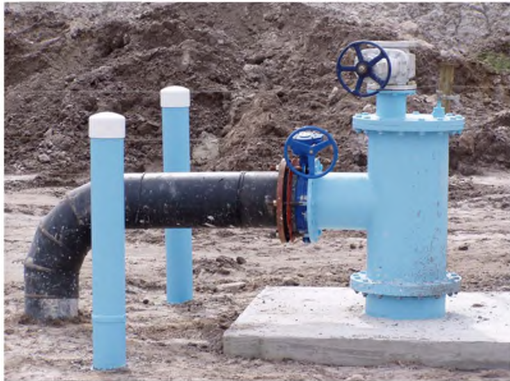
Figure 6. Photograph of MF-41 wellhead.
