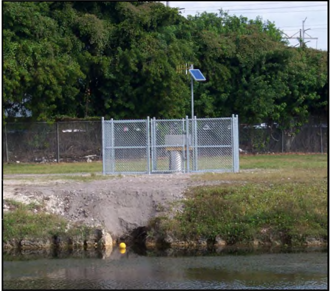
Figure 10. Instrumented surface water monitor station.
