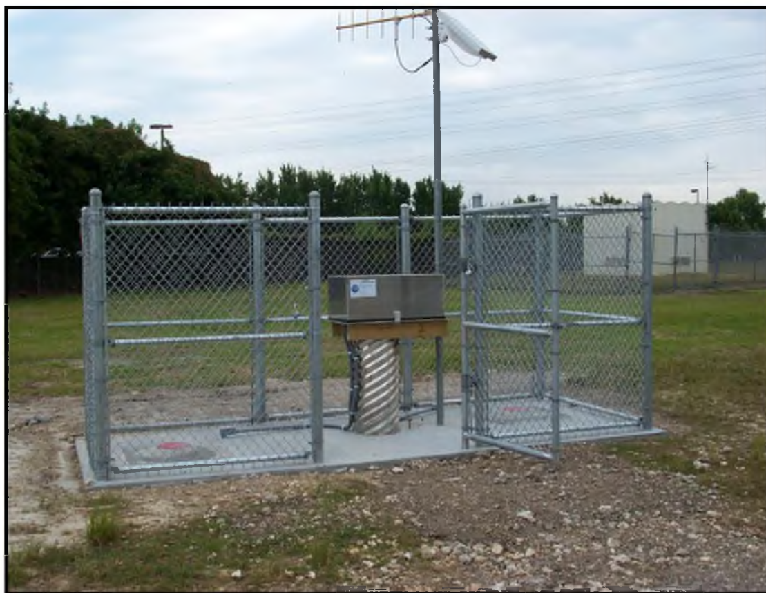
Figure 9. Instrumented groundwater monitor station.
