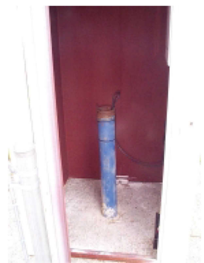
Photograph 1: BF-1 (Lower Floridan Aquifer Well)
