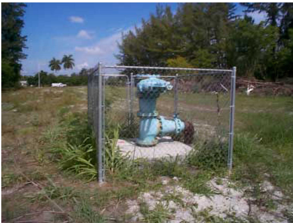
Figure 5. Well PBF-6 Completed Wellhead.
