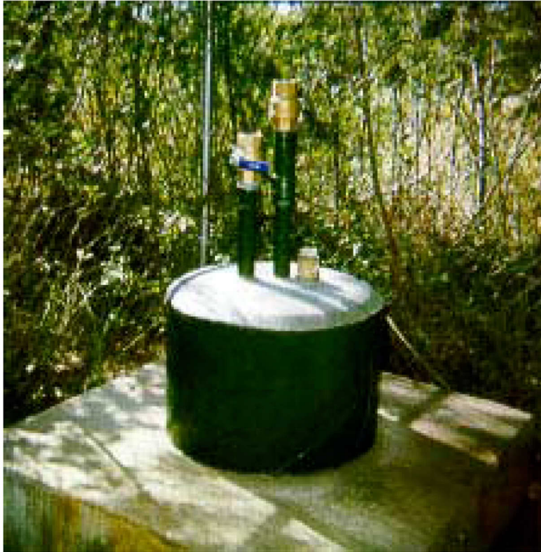
Figure 4. Rebuilt (2001) Wellhead for Wells PBF-3, PBF-4, and PBF-5.
