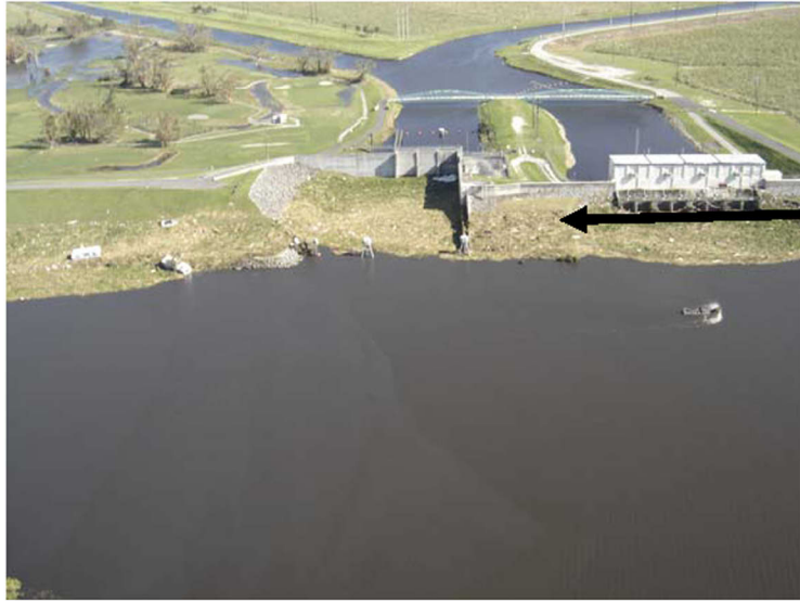
Figure 45. Vegetation pushed into hurricane gate S-351 and pump station S-2 along the south shore of Lake Okeechobee during Hurricane Wilma (photo by SFWMD.)
