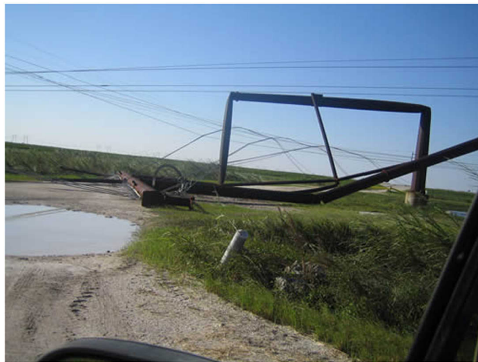
Figure 36. High-power transmission line damage by Hurricane Wilma in an STA (photo by SFWMD).
