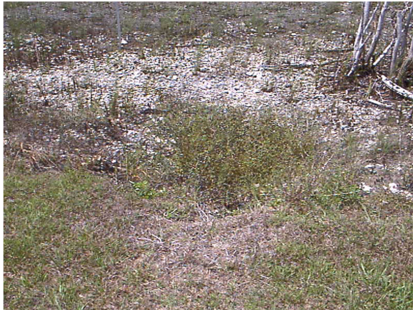
Figure 4 The outlet of Culvert 24 (at the center of the photograph) covered by dense grass
