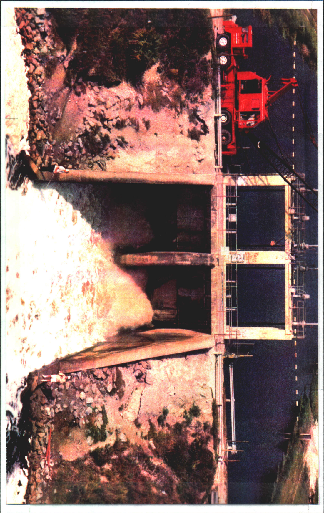
Figure A-2. Gated Spillway S-49 on the C-24 Canal
