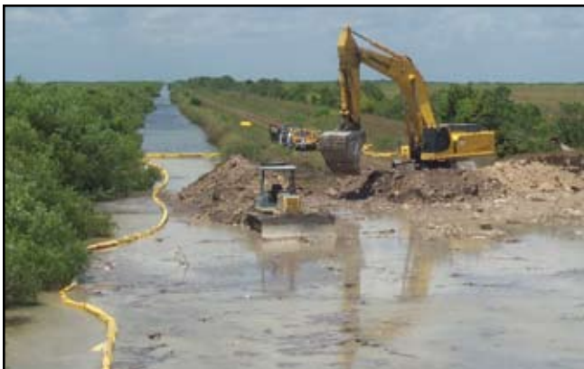
Degradation of the L-67 extension canal and levee. Photo by Elizabeth Crisfield, ENP.
