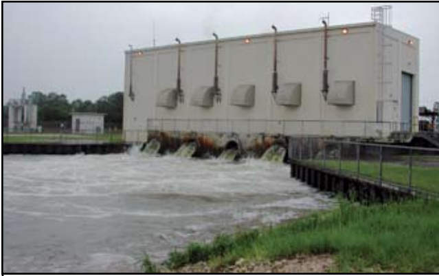
S-332D pump station in the C-111 Project area. Photo by Kevin Kotun, ENP.
