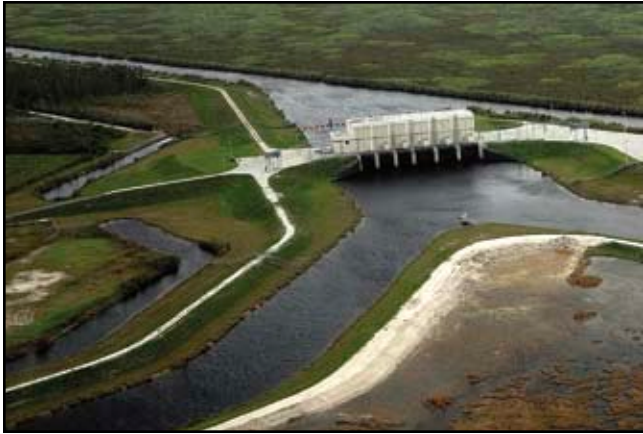
S-362 outflow pump station from STA-1E on the northeast side of the A.R.M. Loxahatchee National Wildlife Refuge. Photo by William Perry, ENP.
