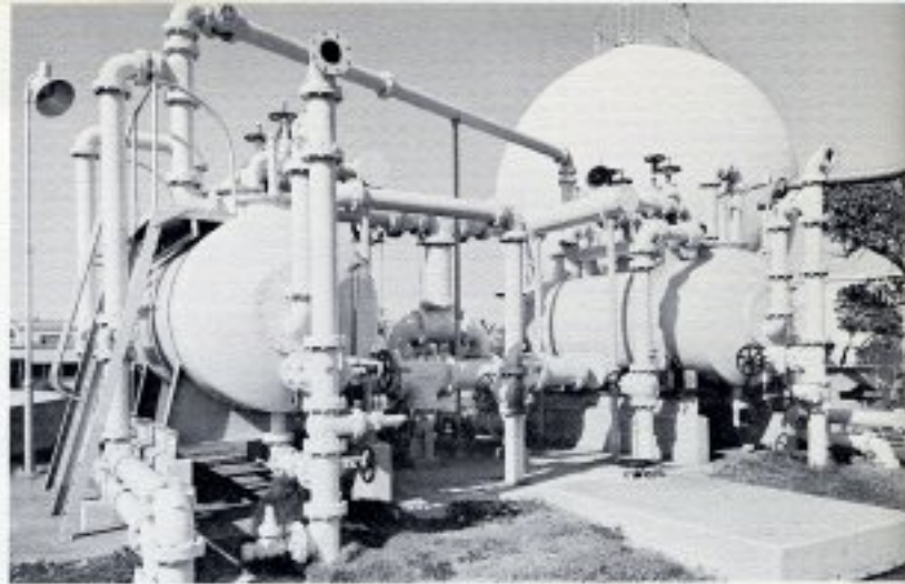
GAS SCRUBBERS reduce sulfides in gases to provide plant fuel.
