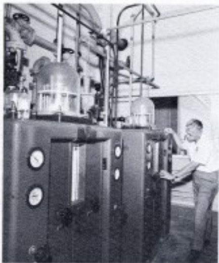
MAKING WATER PURE. To eliminate color, taste, odor and bacteria, chlorine is applied under constant and careful supervision.
