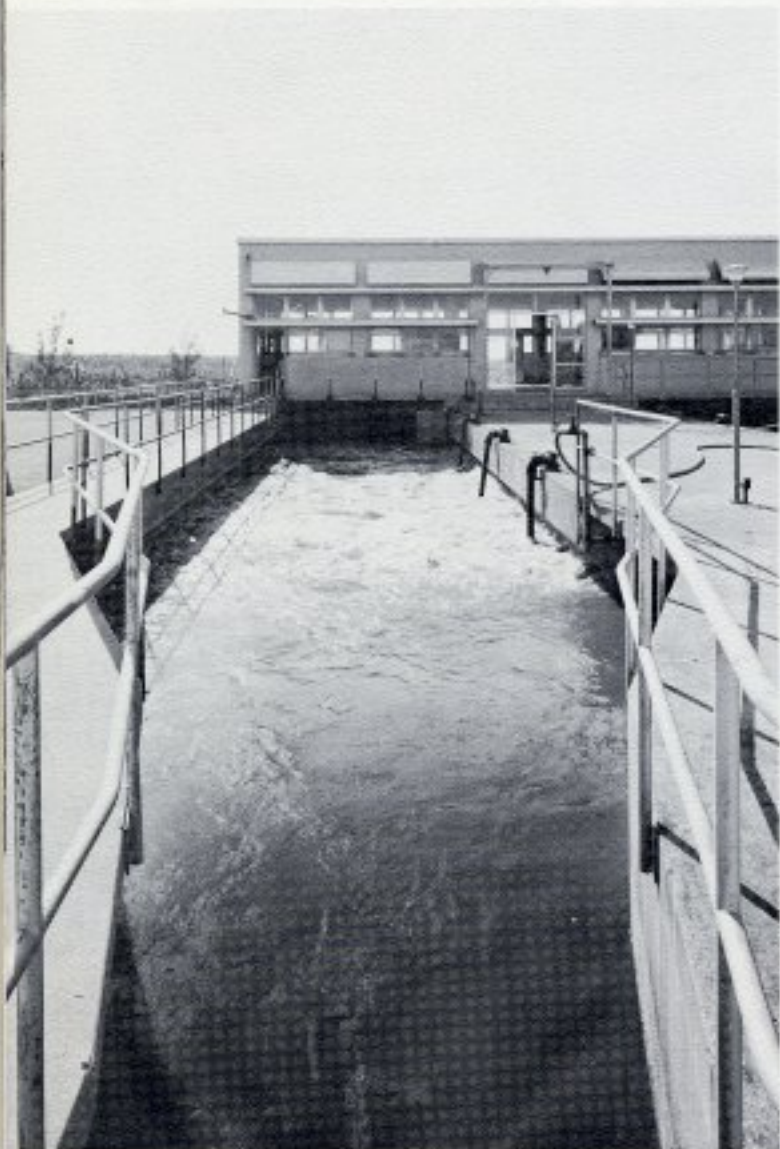
-HERE COMES THE CULPRIT. Raw sewage which formerly caused pollution of Biscayne Bay is now flowing into the grit chambers where sand and other mineral matter are removed, prior to treatment.
