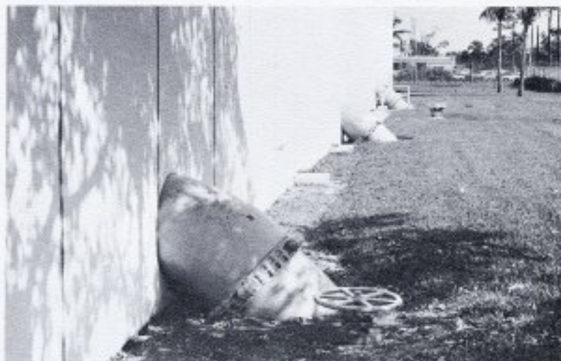
ON ITS WAY. Large transmission mains carry pure water from the treatment plant to the distribution system where "Willing Water" serves your needs.
