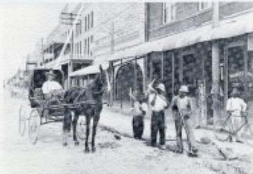
AN EARLY WATER MAIN installation by pick and shovel in Flagler St. and 1st Ave. in the year 1913.
