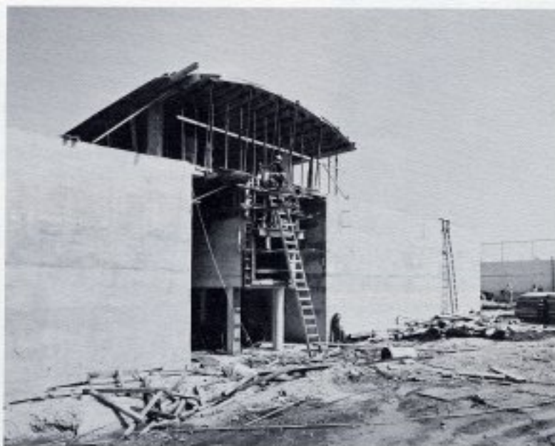
MORE CLEAR WATER. Completion of the construction of the filters for the John E. Preston Plant will provide the customary pure, clear, softened water.
