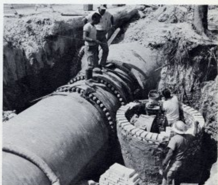
THE OLD AND THE NEW. The Hialeah Treatment Plant, originally built in 1925, will be interconnected to the John E. Preston Plant of 1966 through pipes such as these.
