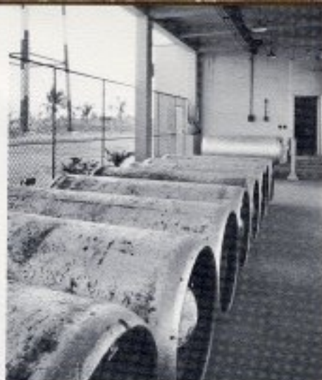
CHLORINE — THE PURIFIER. The addition of chlorine is continually applied at several points.
