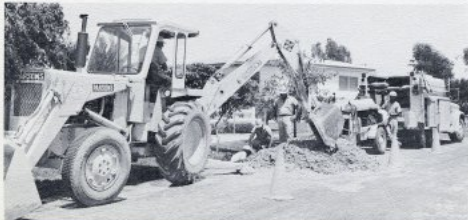
SERVICE TO A CONSUMER. Mechanical equipment is used to install a service pipe between the water main in a street and the consumer's property line.
