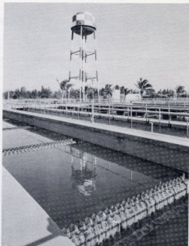
CLEAR AND CLEAN. The final effluent from the plant is inoffensive as it leaves the final settling tanks ready to be chlorinated.
