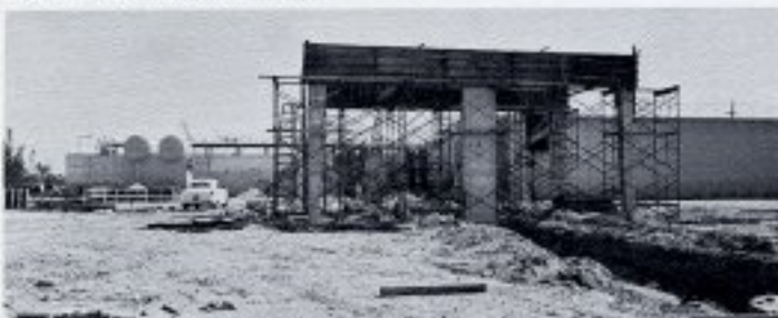
John E. Preston Water Treatment Plant
