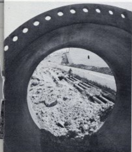
SIX FOOT PIPE. In the construction of the John E. Preston Treatment Plant, pipes up to 72-inches in diameter have been installed.
