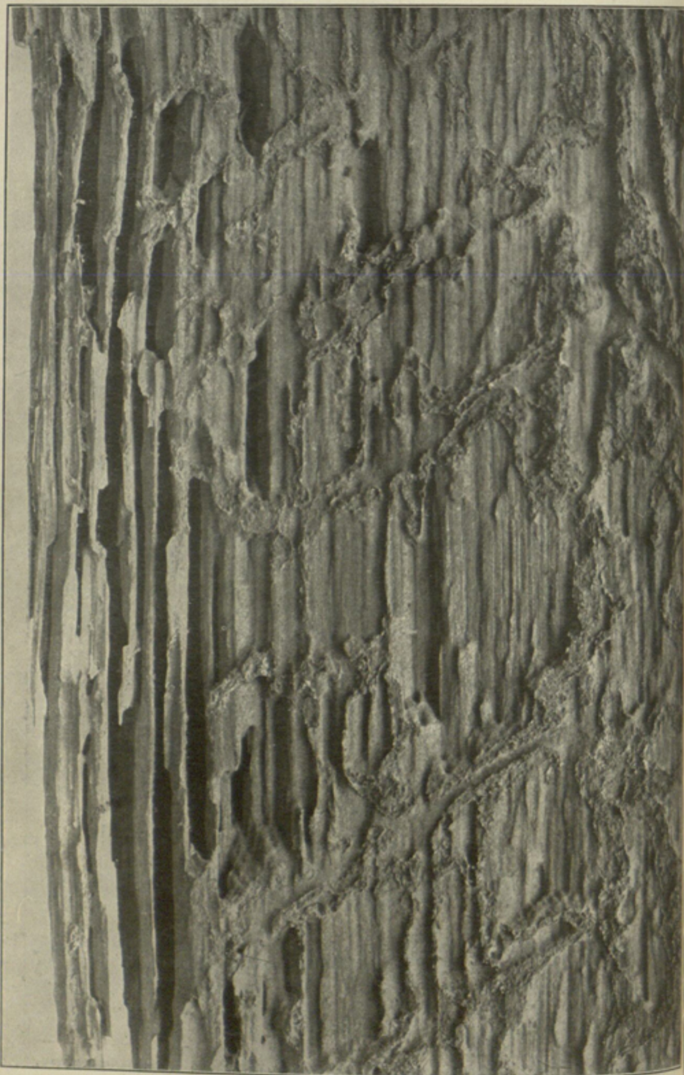
DOOR CASING OF SOUND OAK TIMBER RIDDLED BY WHITE ANTS ( LEUCOTERMES ), SHOWING RUNWAYS COATED WITH EARTH AND EXCRETED WOOD.
