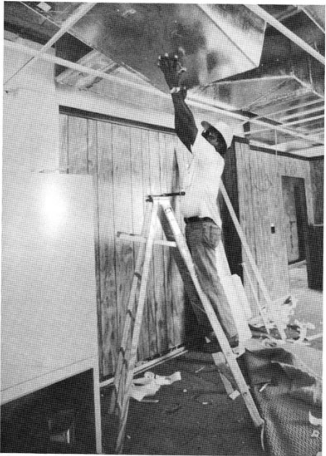
Contractors receiving training and group support from Allied Minority Contractors, a group of professional Black contractors, made renovations to The Business Assistance Center.
