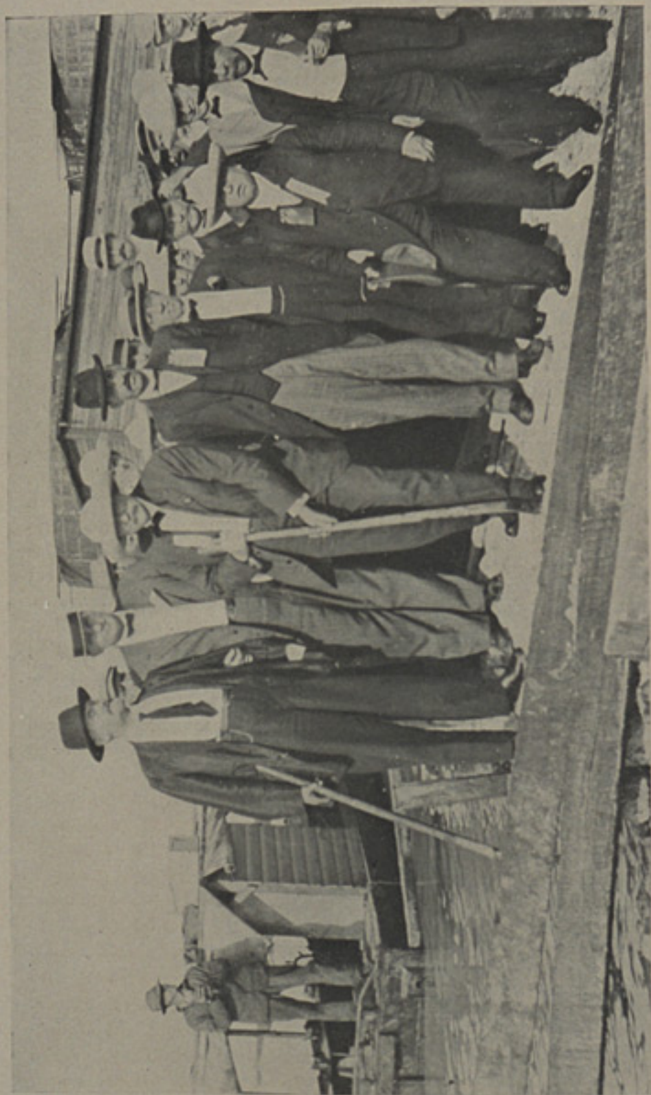
GOVERNOR GILCHRIST TURNING THE WATERS OF THE GULF INTO THE ATLANTIC North Lauderdale Canal, April 25th, 1912
