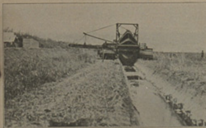
Ditch running parallel to State Canal on Davie Farm. This ditch will be considerably enlarged by a suction dredge and converted into a collection canal.
