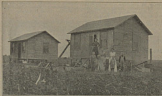
Two Cottages Being Built by the Hill Brothers on Everglade Muck, Davie Experimental Farm. These Houses Are to Be Finished on the Outside With Cement Plastering. Many Buildings Are Now Being Constructed on the Davie Farm.
