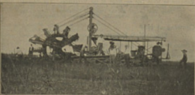
Bockeye Ditching Machine—Property of the Everglade Land Sales Company. This Machine Will Probably be Replaced by a Much Larger Machine of the Same Type for Cutting the Lateral Ditches in the Royal Glade Tract.
