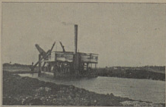
Dredge "Miami," Eating Its Way Through the Muck, Headed for Lake Okechobee.
